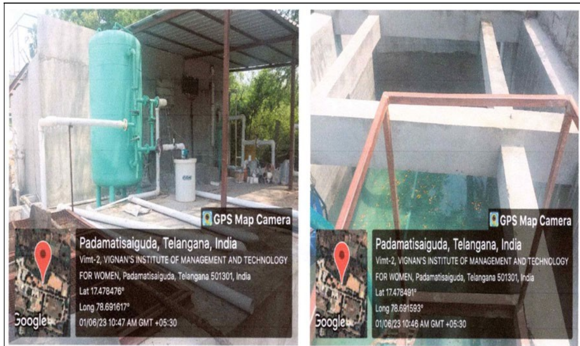
Figure 9.11.10: Sewage Treatment Plant
